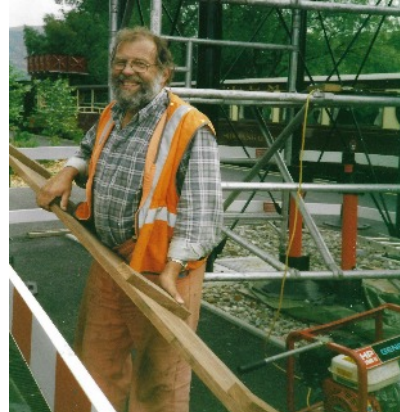
Above - Dave Kent at Waunfawr in July 2001, engaged in building the foot bridge.
